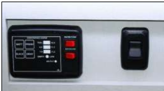
Centralized Monitor/Control Center
