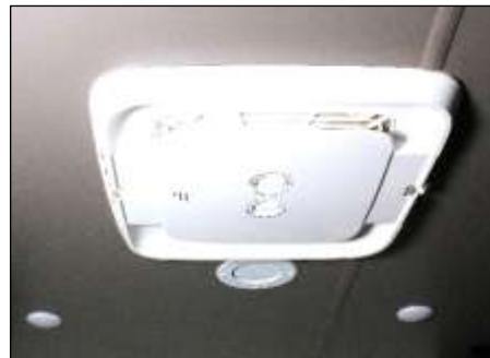
Ceiling-Mounted A/C & Heat Duct
