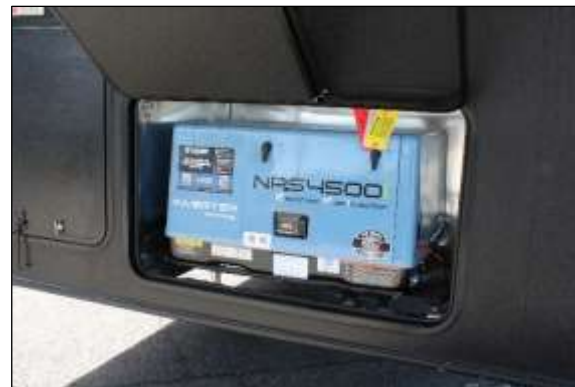
4.5 KW Yamaha Generator
