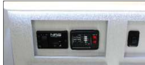
Convenient Monitor & Generator Controls
