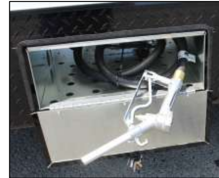
40-Gallon Fuel Station
