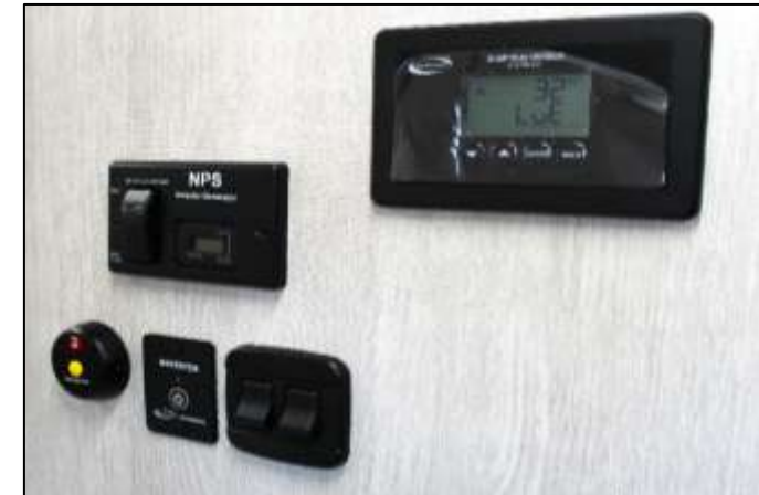
Convenient Solar & Generator Controls
