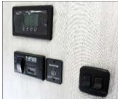
Inverter/Generator Control Center
