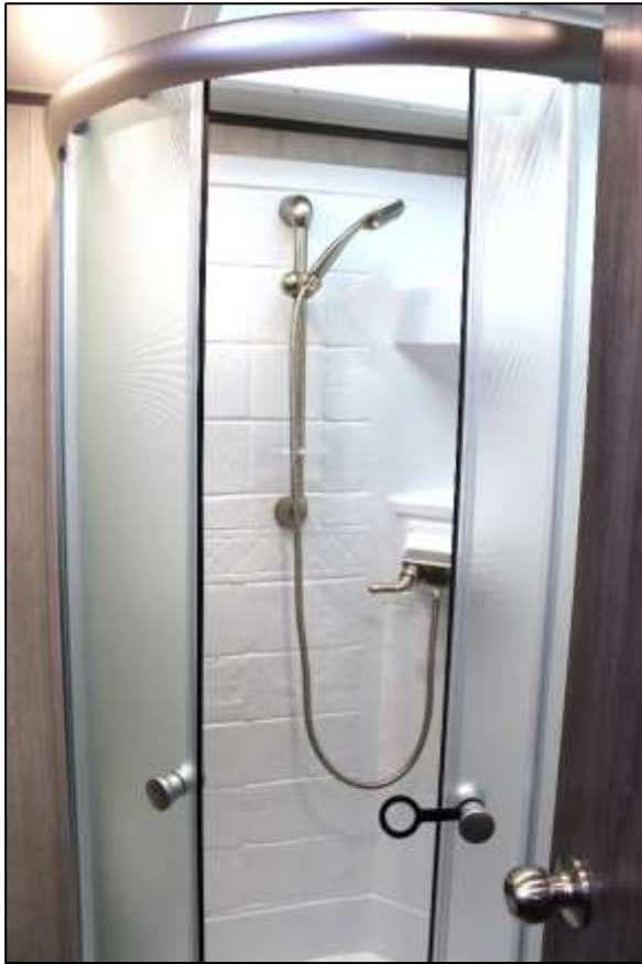
Fiberglass Shower w/Glass Door & Overhead Skylight
