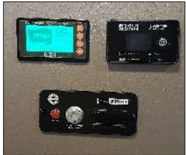
Inverter/Generator Control Center
