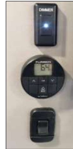
A/C & Lighting Controls
