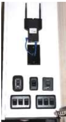
Centralized Control Center
