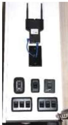
Centralized Control Center
