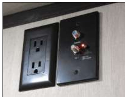
TV Ready – 110v, Cable & Antenna Hookups
