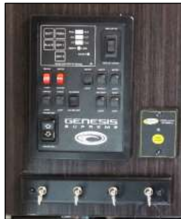
Central Monitor/Control Panel
