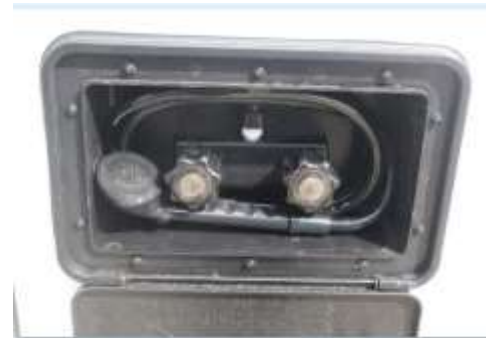
Exterior Shower w/ Hot & Cold
