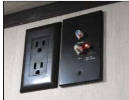
TV Ready – 110v, Cable & Antenna Hookups
