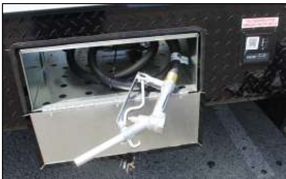
40-Gallon Fuel Station
