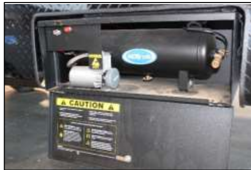
On-Board Air Compressor
