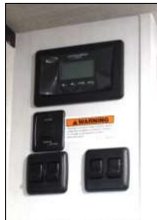
Solar, Awning & Lighting Controls
