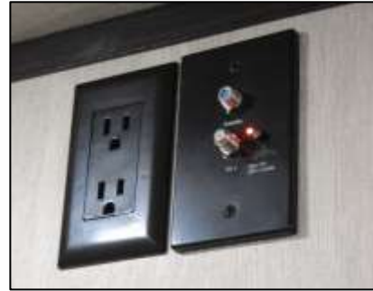
TV Ready – 110v, Cable & Antenna Hookups
