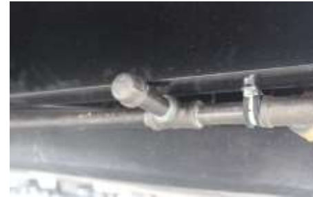
Plumbed for Exterior Propane
