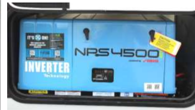
Yamaha 4.5KW Generator
