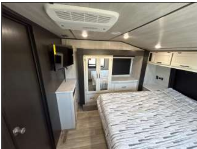
Ceiling-mounted A/C with wall-mounted Controls
