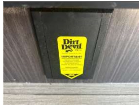
Central Vacuum System
