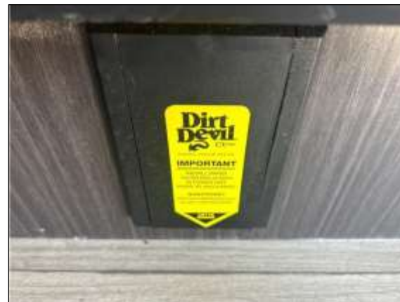
Central Vacuum System
