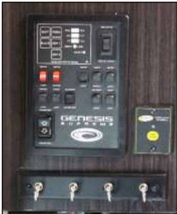
Central Monitor/Control Panel
