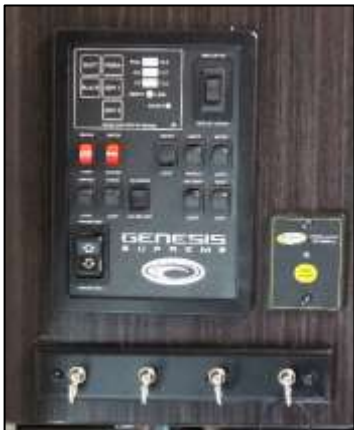
Central Monitor/Control Panel
