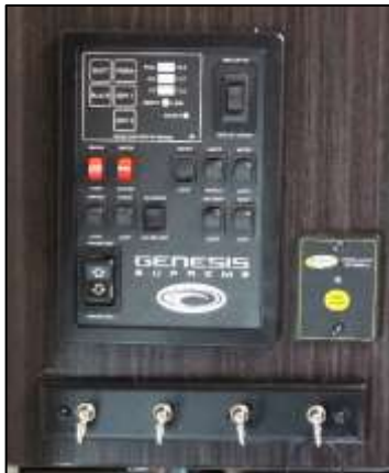
Central Monitor/Control Panel
