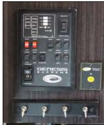
Central Monitor/Control Panel
