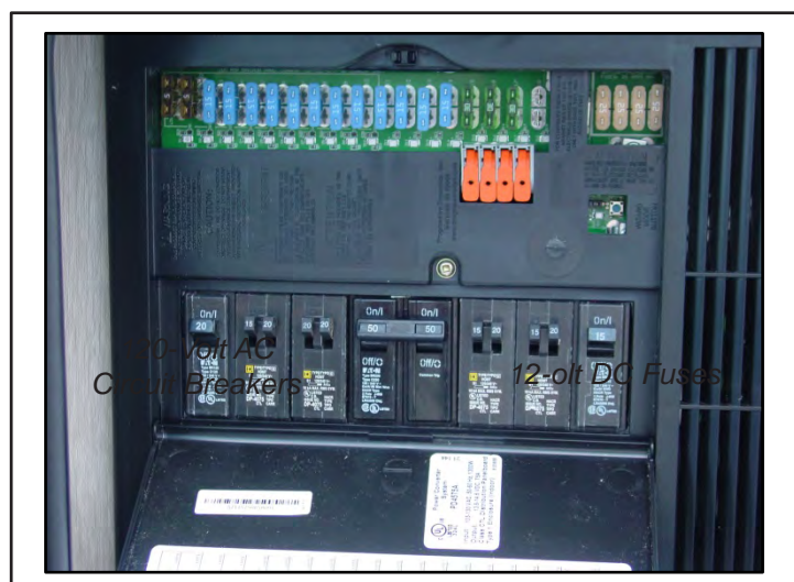
Circuit Breaker and Fuse Panel (Layout varies depending on model)
