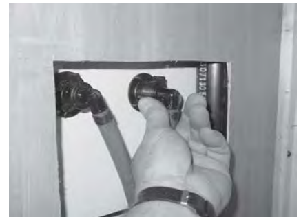
Typical shower/tub faucet fittings
